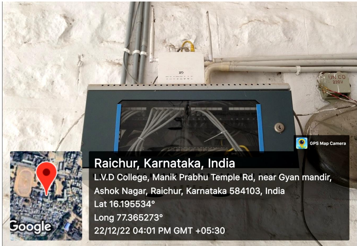
Wi-Fi setup Near Office.
