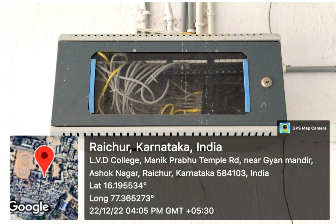
Wi-Fi setup First Floor Near Electronics Department.
