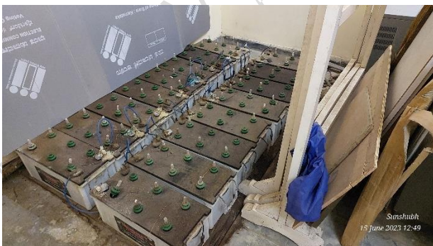
Batteries stacked without ventilation.
