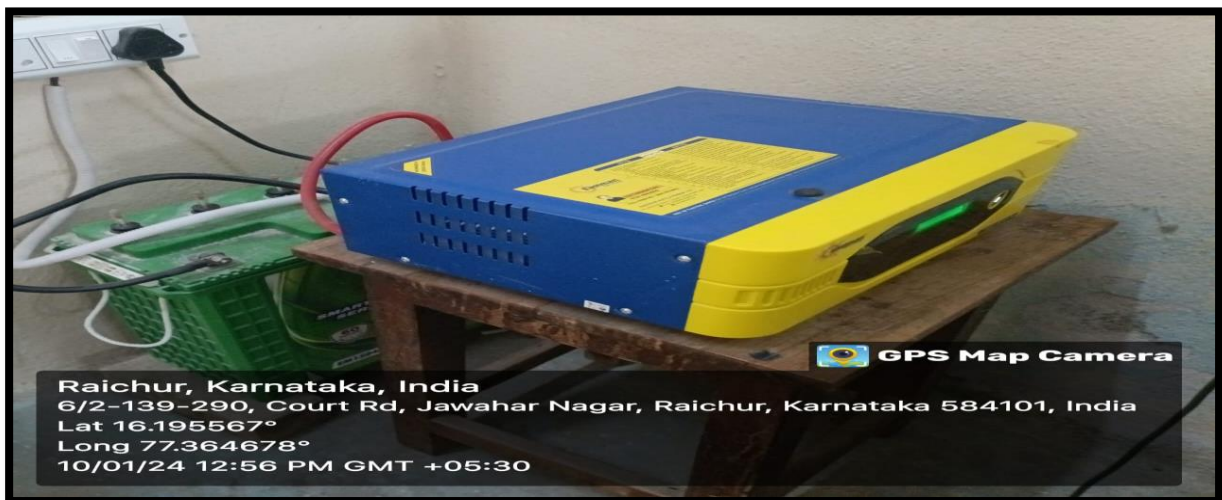
POWER BACKUP IN NAAC ROOM
