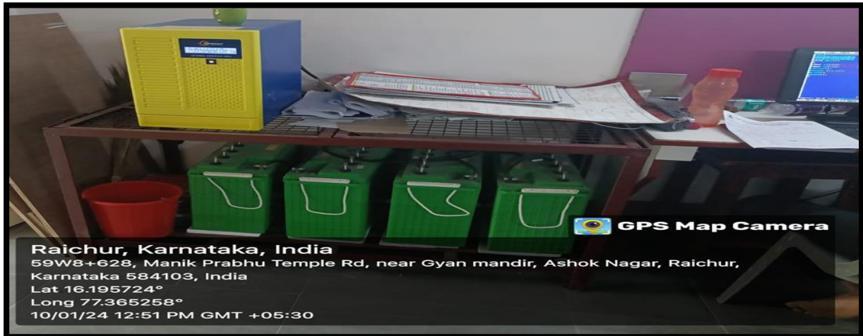
POWER BACKUP IN COMPUTER LAB3
