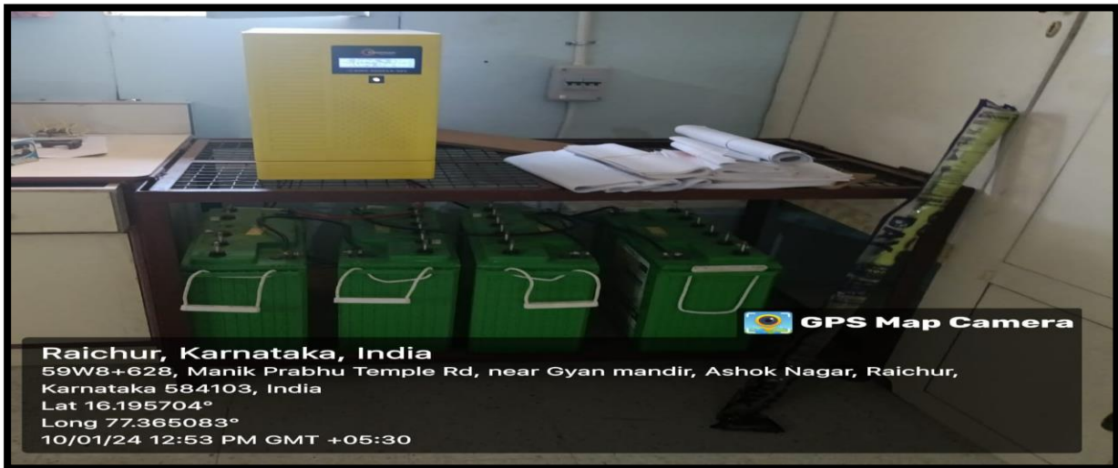
POWER BACKUP IN COMPUTER LAB2
