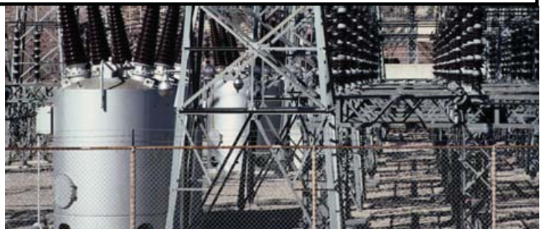
The large cylindrical transformers on the left of this photo convert electricity from 350,000 V to 15,000 V at an electrical substation.
