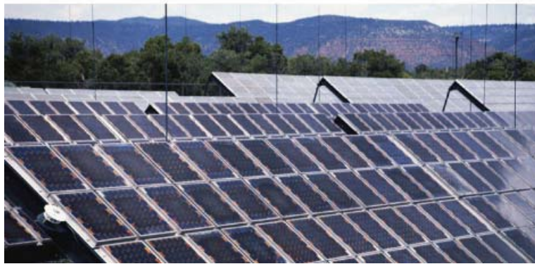
Banks of photovoltaic cells populate a "solar energy farm" that can produce hundreds of kilowatts of electric power.
